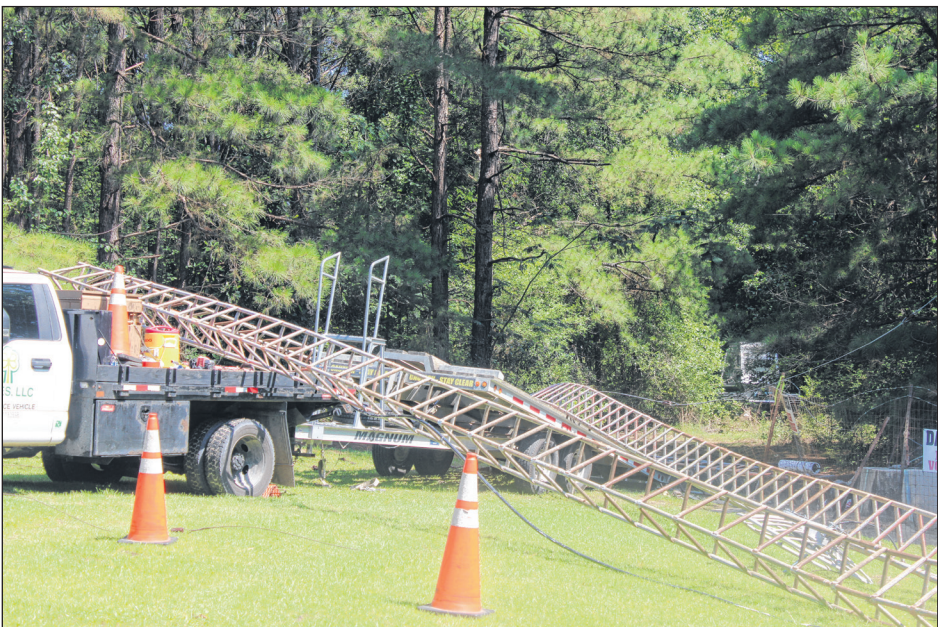
The WLNC broadcast tower rests on a vehicle belonging to a tree removal company after collapsing during work at the station's Lila Drive location. The collapse knocked WLNC off the air.
