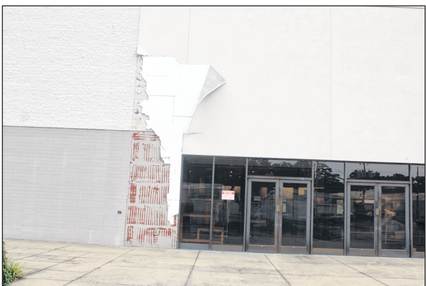
Winds tore the siding off of the Belk store at Biggs Park Mall in Lumberton during a thunderstorm on Friday.
