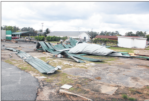
A structure at the corner of North Cedar and East 21st streets in Lumberton was damaged by straight-line winds during a thunderstorm on Friday.
