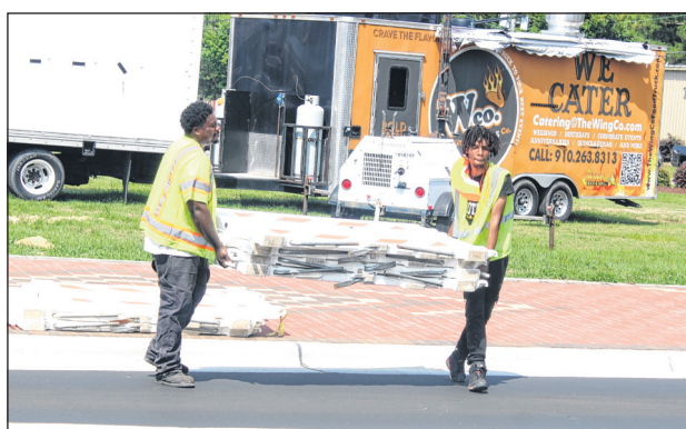
Chris Stiles | The Robesonian Construction workers move barricades after Third Street in downtown Pembroke reopened on Friday following a 10-month closure.
