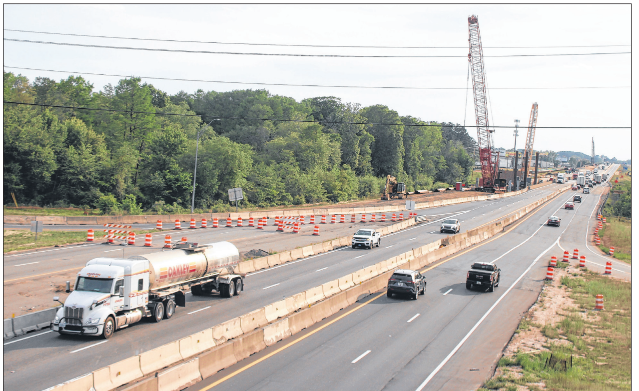
Chris Stiles | The Robesonian Motorists travel along Interstate 95 near exit 19 in Lumberton on Monday, as cranes and other construction equipment sit on the roadside as part of the project to widen and elevate the highway.
