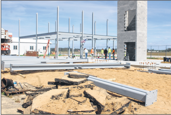
Tomeka Sinclair | The Laurinburg Exchange Construction continues Thursday on the new 8,200-square-foot terminal at Laurinburg-Maxton Airport. The two-story terminal is expected to feature expansive glass, a vaulted lobby ceiling and entrances from both the roadway and the airfield. An interior overlook will provide clear views of the runway, taxiway and arriving aircraft.
