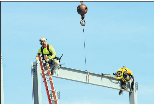
A steel beam is lifted into place Thursday during construction of the new terminal at Laurinburg-Maxton Airport. Officials marked the moment as a key milestone in the project.
