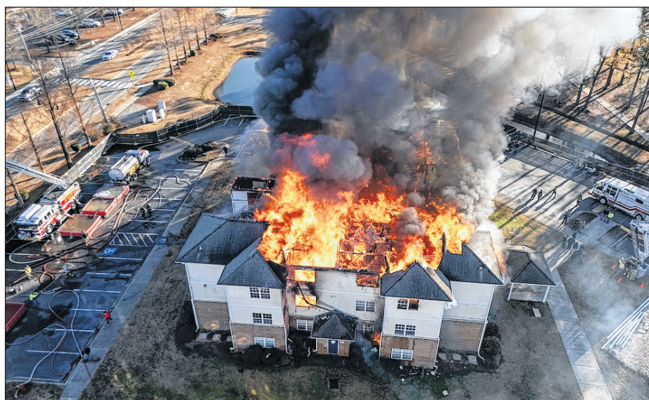
Photos courtesy of UNCP A controlled burn at the Village Apartments on the UNCP campus. The six buildings in the complex were demolished by controlled burns between Dec. 21, 2024, and Jan. 5, 2025.
